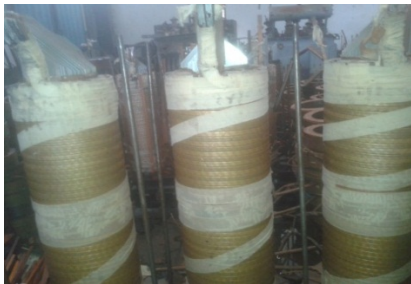
Fig. 2 LV Coil Inspection
