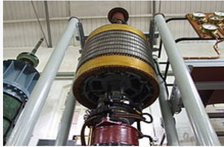
Fig.5 Rotor of a large water pump. The slip rings can be seen below the rotor drum.
